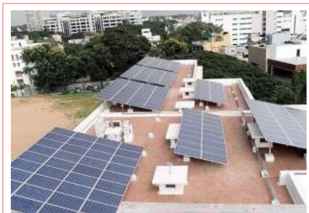
Installed Solar Panels at Surangi Unit, reducing 80 MT carbon emissions per month
