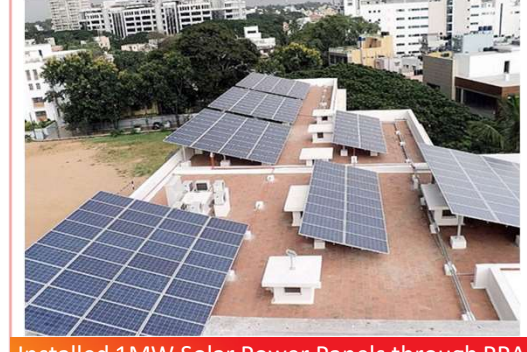
Installed 1MW Solar Power Panels through PPA with Amplus Solar, the installed capacity now stands at 1.7MW
